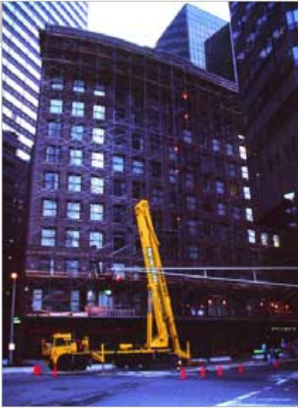
Installation was handled by Marr Scaffolding, the company used for the renovation. Joanne Rose of the Reno, Nev.-based Impact Imaging serve as a consultant.
