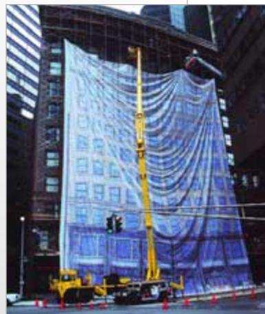
Because of the windy location and the sheer size of the print, Marr opted to involve a professional engineer who calculated the wind load and advised the company on tie-ins for the project.
