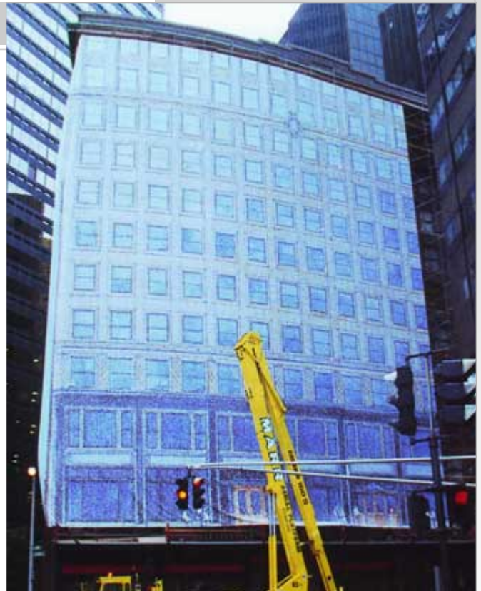
The actual installation took about 10 hours to complete, using a 10-person crew. The image is attached to the scaffold utilizing a mix of threaded connectors, carabiners and ratchet straps.
