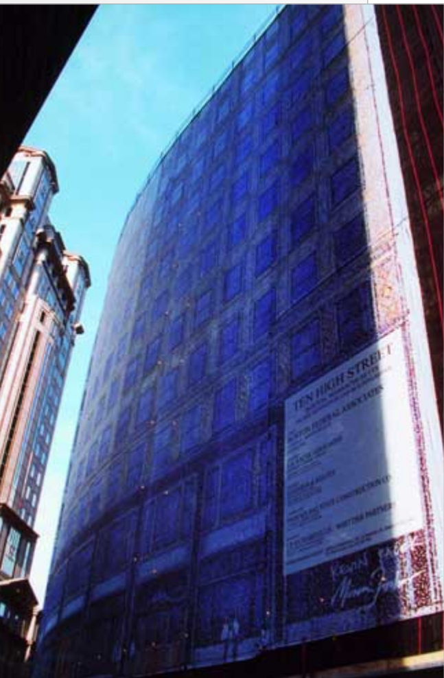
The 11-story, 90,000-square-foot facade of a Boston office gets covered with a stylized print during an upgrade of the building. The pixelated graphic of the finished facade was used instead of the more traditional debris netting required by OSHA.
