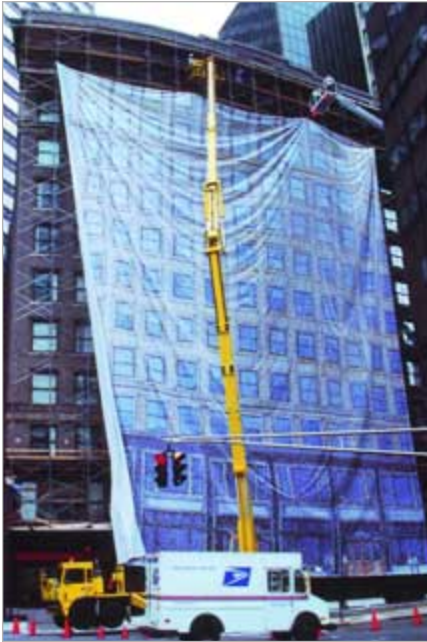
Two 150-foot truck-mounted aerial platforms were employed to lift the folded material to the top of the scaffolding. The largest single piece of the image measures 90 feet in width. It was accomplished without a single tear or rip.
